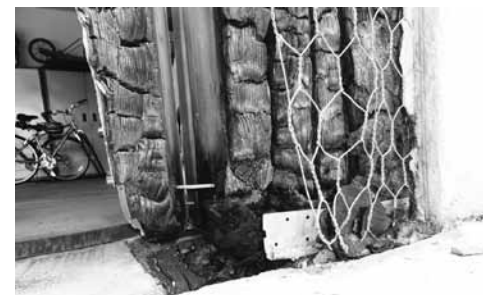
Interior ignition as shown here can be difficult for firefighters to spot during a wildfire. Above photos provided by Insurance Institute for Business & Home Safety.
