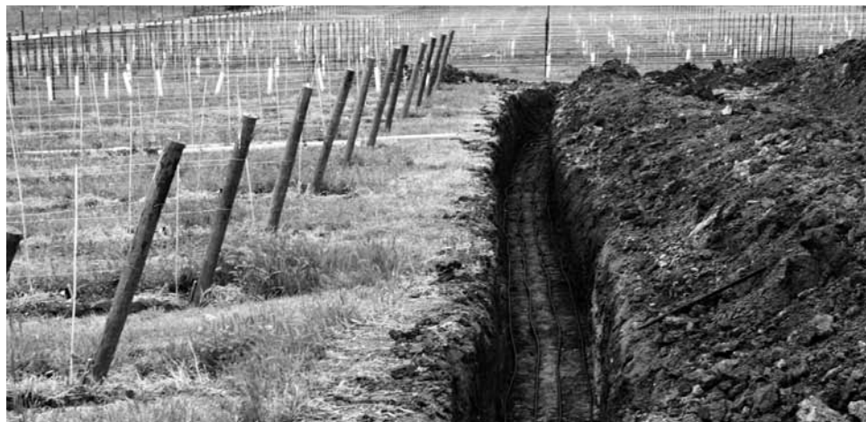
Advanced Air & Metal installed this geothermal system with a horizontal loop at a Rogue Valley vineyard.
