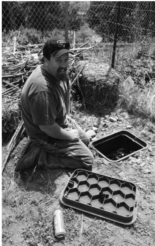
Photos (top) Joshua Morrison helped design and install the new irrigation system. (bottom) Tyler Van Buskirk used a trenching machine from his own business.
