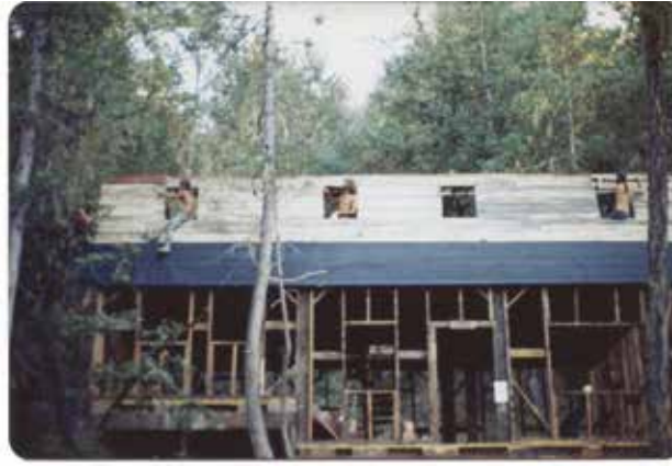
The "Big House" under construction at Molto Bene. Photo courtesy of Mike Kohn.
