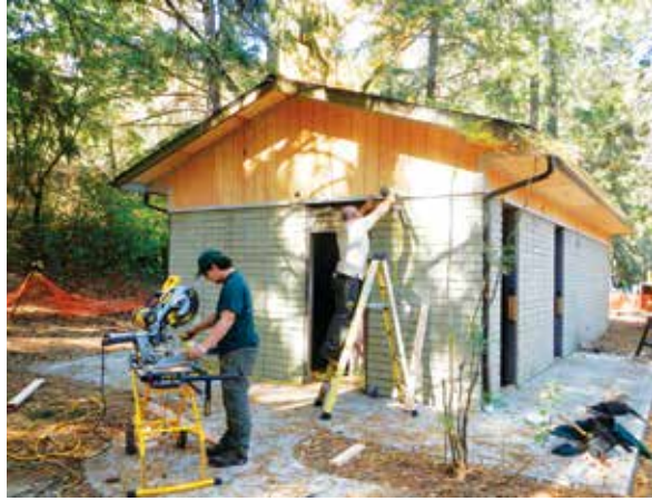
Jackson County Park Rangers Jonathon Bernhardt and Dustin Stafford at work on the day-use restroom. (Photo: Tom Carstens.)
