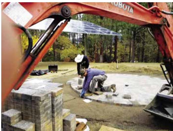
Contractor Francisco Contreras lays the sundial pavers, while his employee Jose assists.
