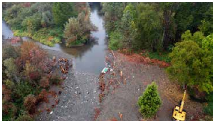
This shows the project site during construction. The dam has been removed and the irrigation headgate has been installed. The bare area on the right shows where gravel has been dug each year to build the pushup dam. This area will revegetate slowly over time. Photo: APWC.
