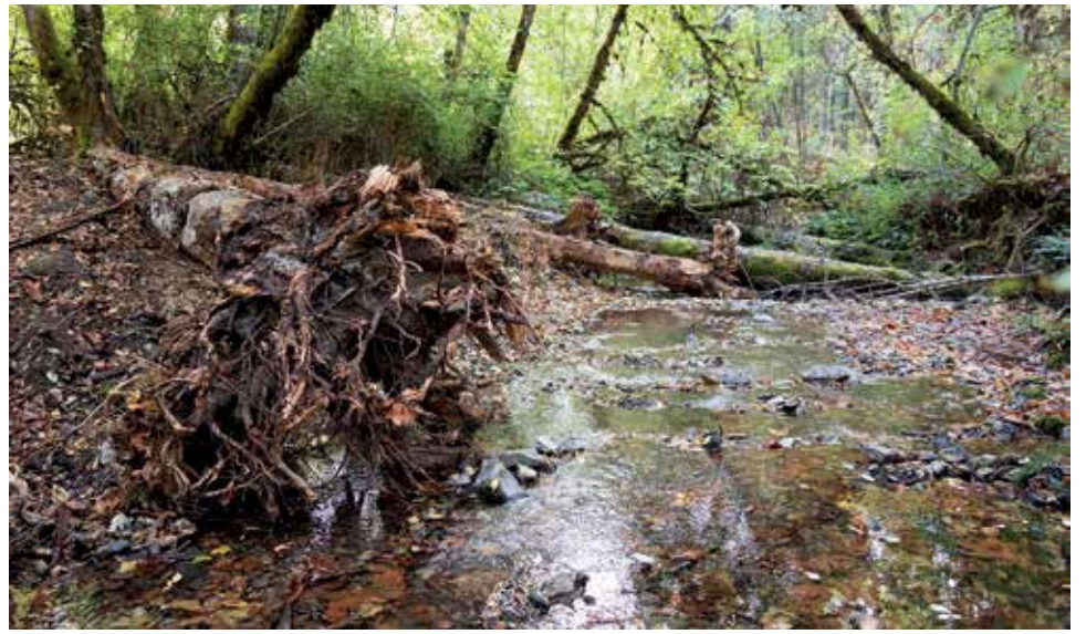
APWC crews placed logs on the floodplain in an effort to reconnect it to Cheney Creek.
