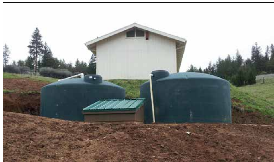
A 10,000-gallon rainwater collection system.
