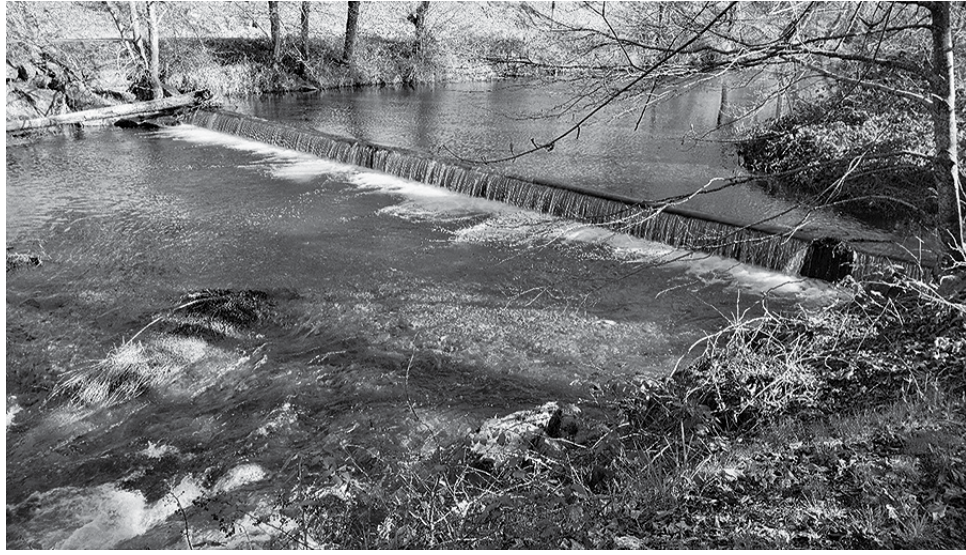
Watts Toppin Dam, on Williams Creek just downstream of the Powell Creek convergence. Photo: APWC.
