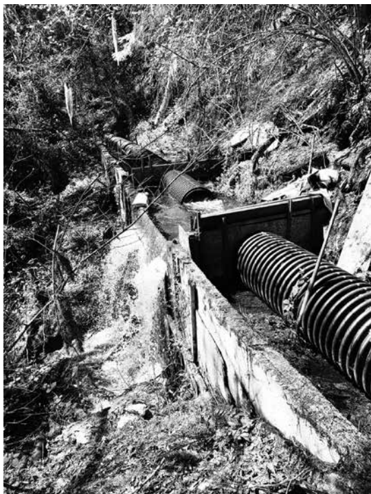
Weir located on the O'Brien ditch. The concrete work dates back to the 1930s. Photo: David Dobbs.
