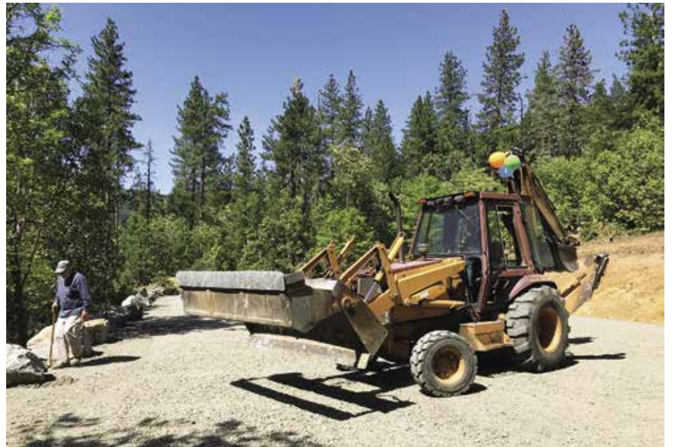
Trailhead construction was completed in mid-May, except for the asphalt approach off Highway 238. Pictured, left to right, Duane Mallams, ATA volunteer, and Roarke Ball on his backhoe with celebratory balloons. Photo: David Calahan.
