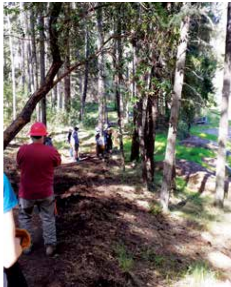
Students working on the trail after learning how to use the proper tools to angle the backslope, find the hinge point, and do the tread with a 3-5 percent outslope. The instructor, Duane Mallams (red hard hat), observes their progress.
