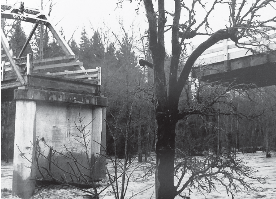
Flood-damaged Applegate Bridge in December 1955, near the mouth of Slate Creek. Photo: Josephine County Historical Society.
