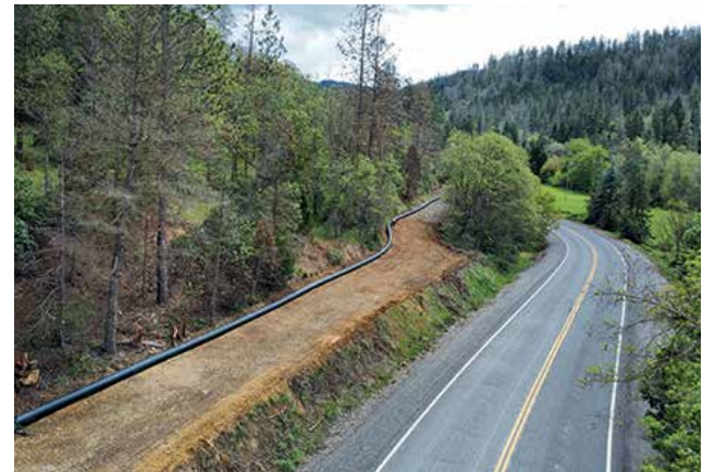
Irrigation pipeline ready to be buried along Little Applegate Road. Photo: APWC.
