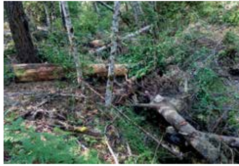
A recently installed LWD structure in Cold Creek illustrates the messiness of stream restoration. Photo: Luke Wimmer.
