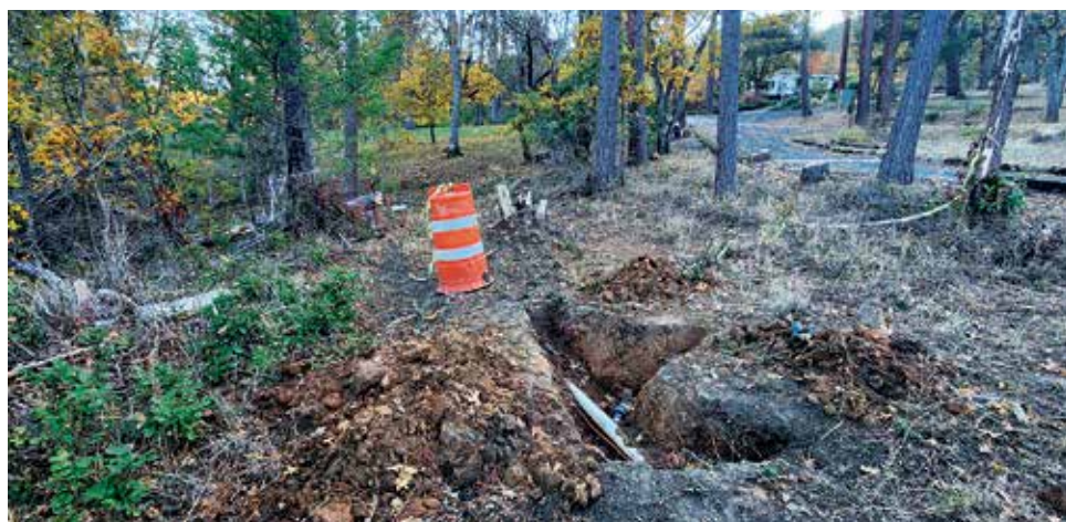
Park personnel are in the process of opening up valve intersections and replacing electric valves with air-pressure valves. Photo: Janelle Dunlevy.
