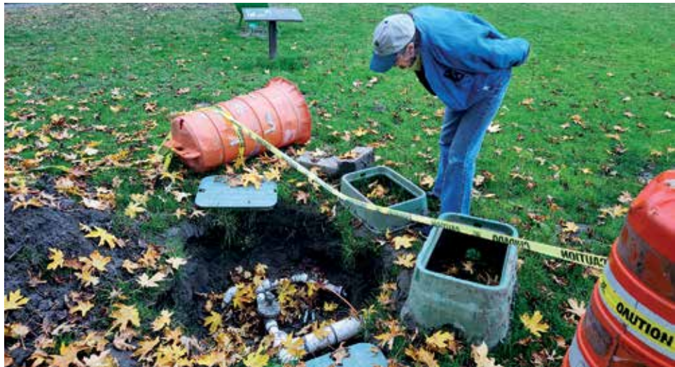
Janis Mohr-Tipton, APWC volunteer park enhancement committee chair, examines the work needed to replace the large valves for the eight-inch pipelines required for irrigation. Photo: Janelle Dunlevy.
