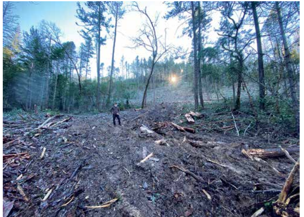
This was a seasonal stream, but BLM logging operations completely filled in the stream channel and converted this small seasonal stream into a skid trail. The clear-cut slope above is unit 27-3. Photo: Luke Ruediger.
